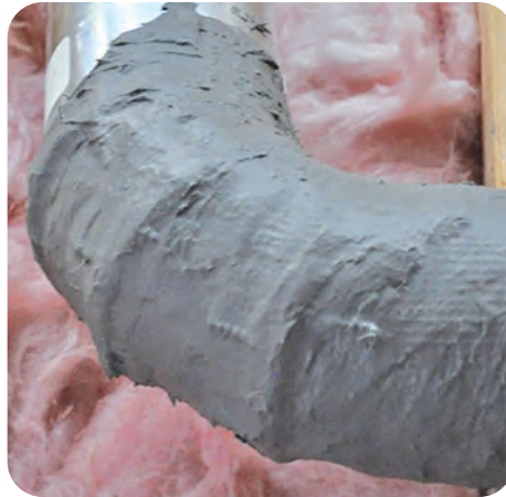
A-2. Apply mastic over all mesh tape and all gaps, seams, joints, etc.
